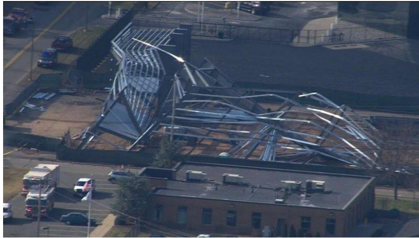
A steel framed hanger building that collapsed during construction
