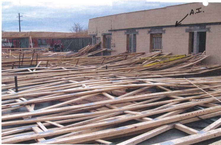
Wood trusses that collapsed during construction
